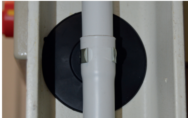
Fastening empty conduits or cables directly to steel beams
